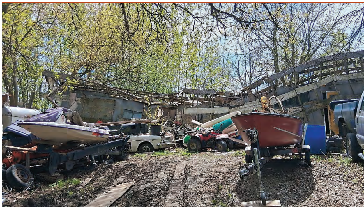
Photo 28. View of a collapsed construction trailer or storage shed.
