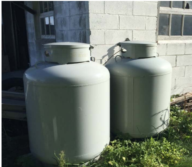
Photograph 3. View of propane tanks outside the workshop at 5584 Lakeshore Road. (Septembe r2016)
