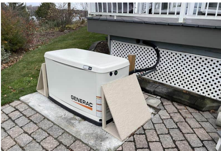
PHOTO 5: View of the natural gas powered back-up generator located adjacent to the residential dwelling, facing northeast.
