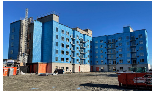
ABOVE: Progress shown of the northwest elevation of Mosaic House. Photo provided by York Region.
