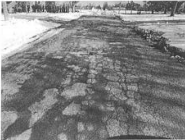
Photo 1: Edward Street looking north, showing severe alligator cracking, severe distortions, severe ravelling, and moderate potholes
